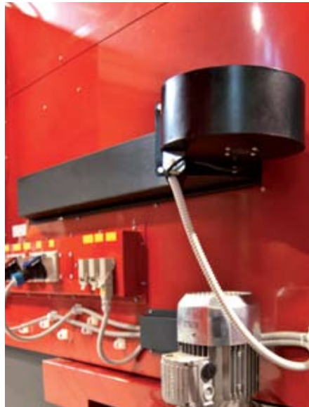
Electric control panel
